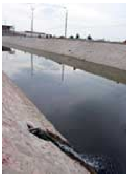
Untreated wastewater discharged into To Lich River
